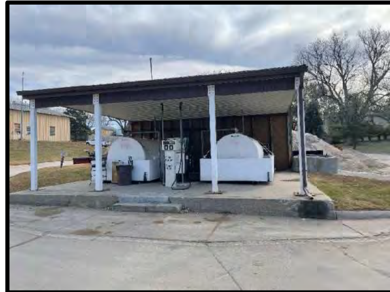
Picture 24: Covered Fueling Area – 11/14/2023
