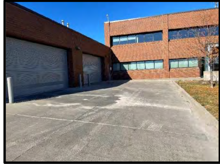
Picture 18: Trackout From Vehicle Washout Garage – 11/21/2023
