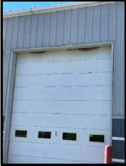
Picture 5: Stains on Garage Door Bay 9 – 10/16/2023
