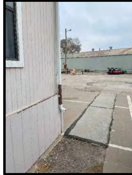
Picture 2: Downspout on SE Corner Street Department Office – 11/16/2023
