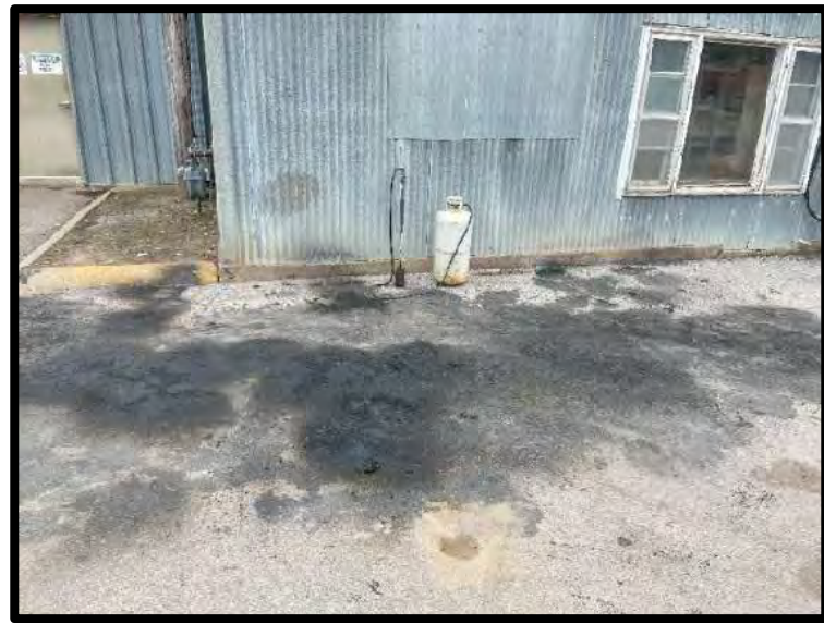
Picture 14: Tar/Asphalt Cleaning Area. Stains on Pavement – 11/16/2023
