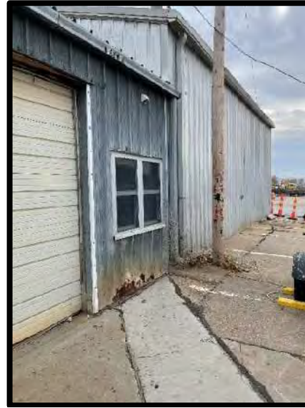
Picture 10: Downspout and Rusting South Side Park Storage Building – 11/16/2023
