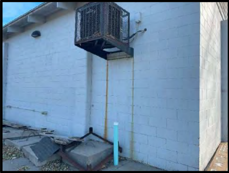
Picture 9: Stains Under Air Conditioner Mount – 11/15/2023
