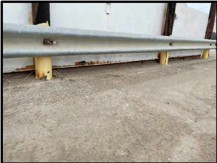
Picture 3: Rusting at Base of East Side Diesel Secondary Containment – 11/16/2023
