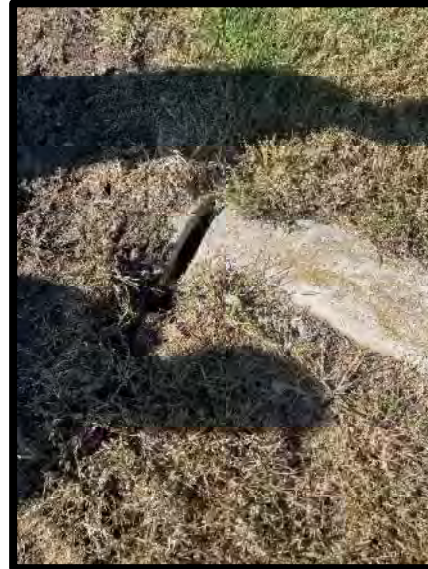
Picture 12: Culvert Inlet Separation Northeast of Facility – 10/16/2023
