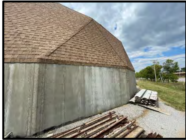
Picture 14: Cracking on Exterior of Salt Storage Building – 9/14/2023
