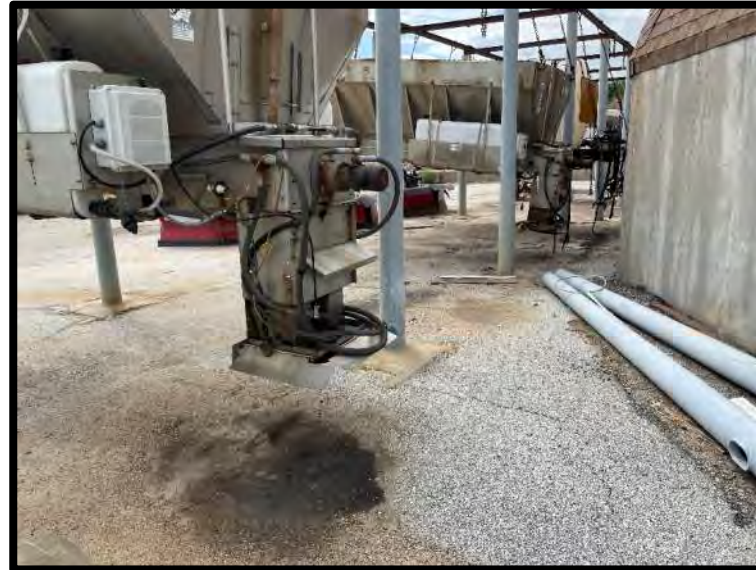
Picture 16: Stains Below Outdoor Salt Spreader Storage – 9/14/2023
