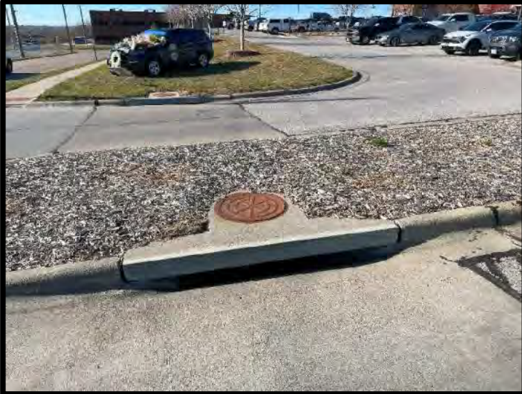
Picture 11: Inlet at Main Facility Entrance – 11/21/2023
