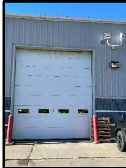
Picture 4: Stains on Garage Door Bay 8 – 10/16/2023
