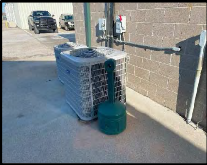
Picture 15: Cigarette Disposal at South Building – 11/28/2023
