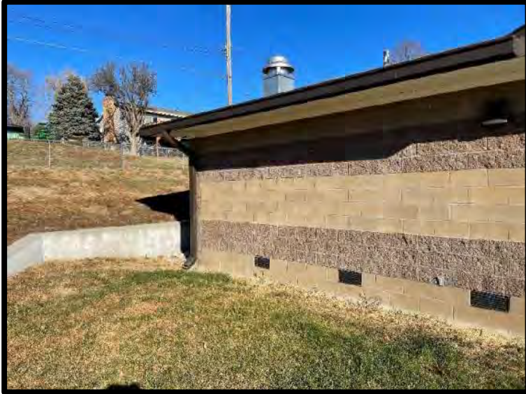
Picture 1: Downspout on Northwest Corner Main Building – 11/21/2023
