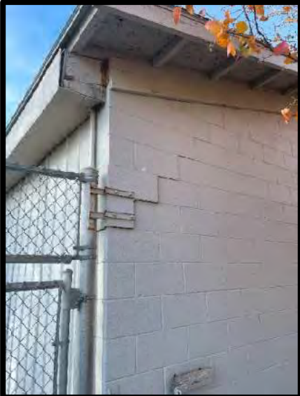
Picture 11: Cracked/Separated Blocks Southwest Corner of Building – 11/15/2023
