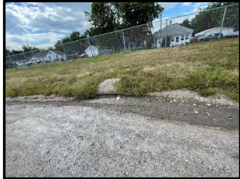
Picture 12: Erosion on Toe of Slope, North Side of Shop – 9/14/2023
