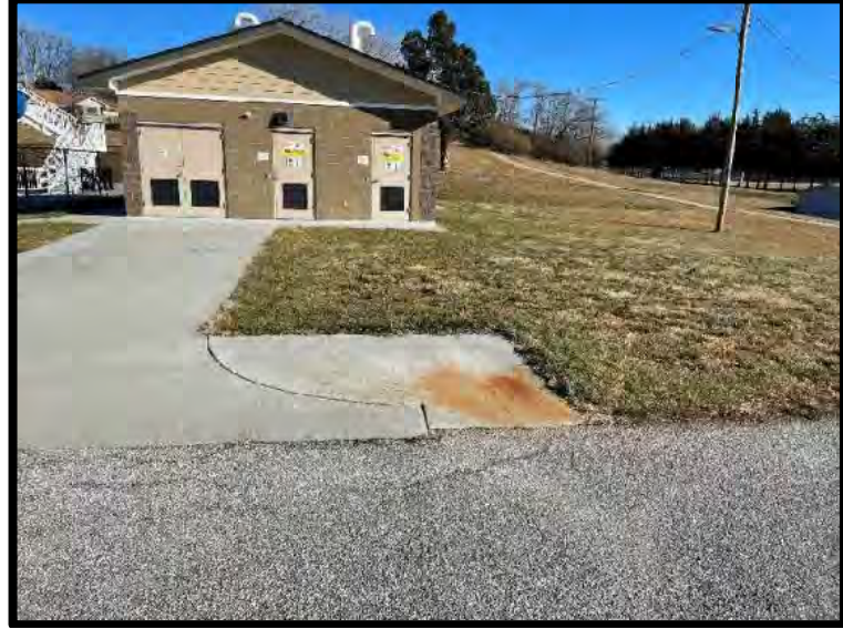
Picture 10: Stains at Dumpster Storage Location – 11/21/2023
