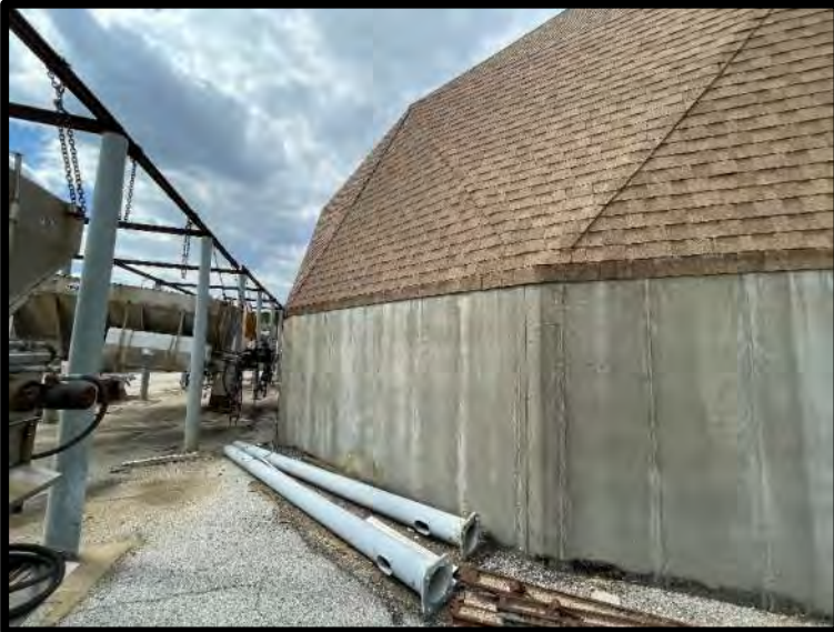
Picture 15: Cracking on Exterior of Salt Storage Building – 9/14/2023
