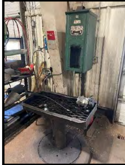
Indoor Used Oil Separator and Oil Filter Crusher – 10/16/2023
