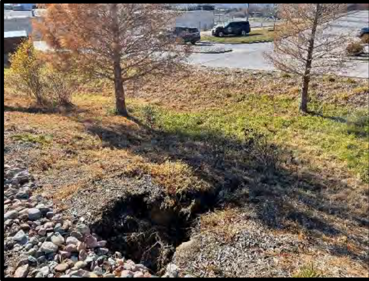
Picture 9: Erosion at Drainage Basin – 11/21/2023
