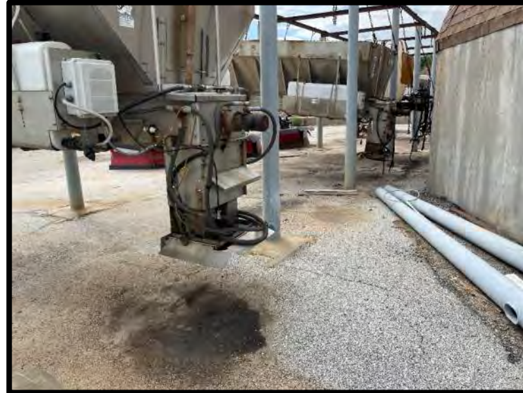
Picture 16: Stains Below Outdoor Salt Spreader Storage – 9/14/2023
