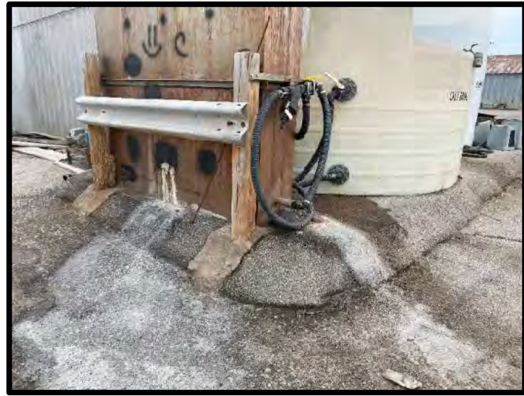
Picture 26: Rusting on Liquid Deicer Mixing Tank – 11/16/2023
