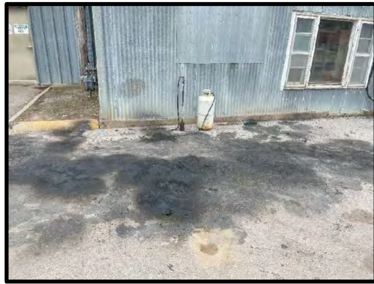
Picture 14: Tar/Asphalt Cleaning Area. Stains on Pavement – 11/16/2023
