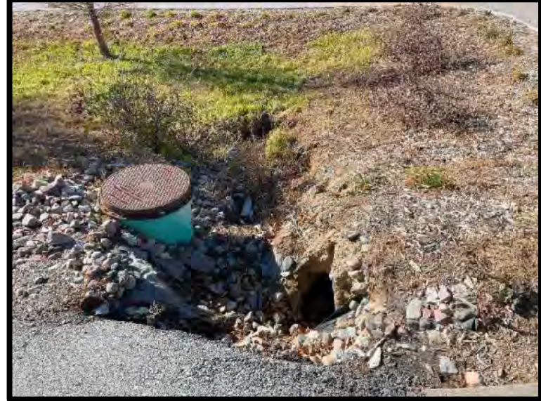
Picture 10: Erosion at Drainage Basin – 11/21/2023
