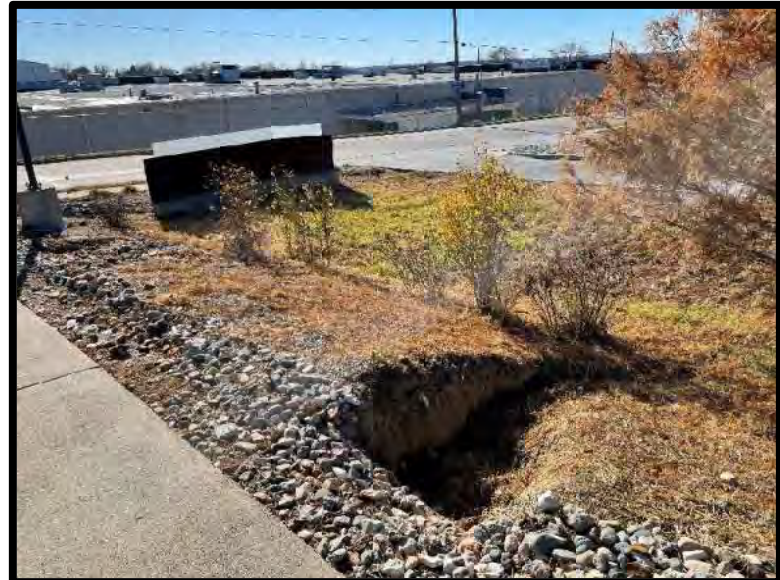
Picture 8: Erosion at Drainage Basin – 11/21/2023
