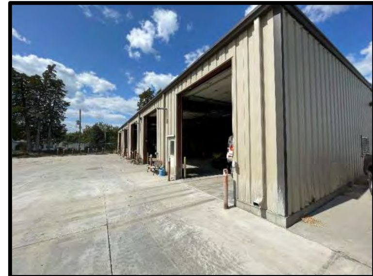
Picture 4: Gutters Drain to Impervious Surface – 9/14/2023
