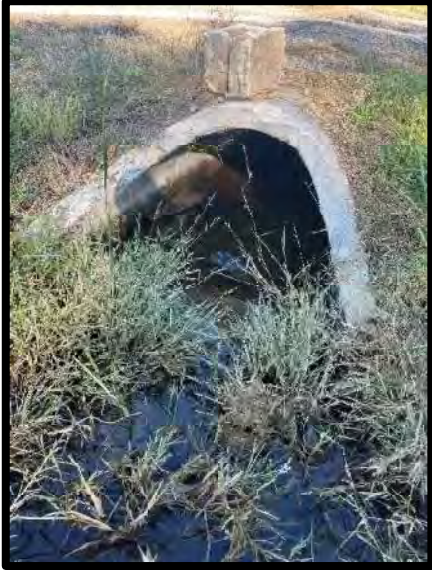
Picture 9: Culvert Outlet Northeast of Facility – 10/16/2023
