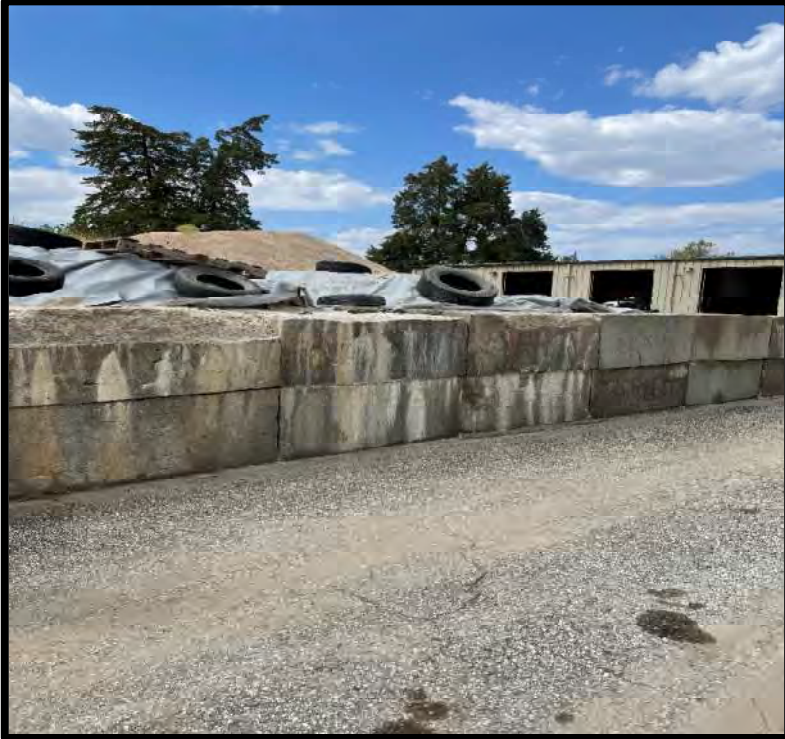
Picture 17: Corrosion on Exterior Wall of Outdoor Storage – 9/14/2023
