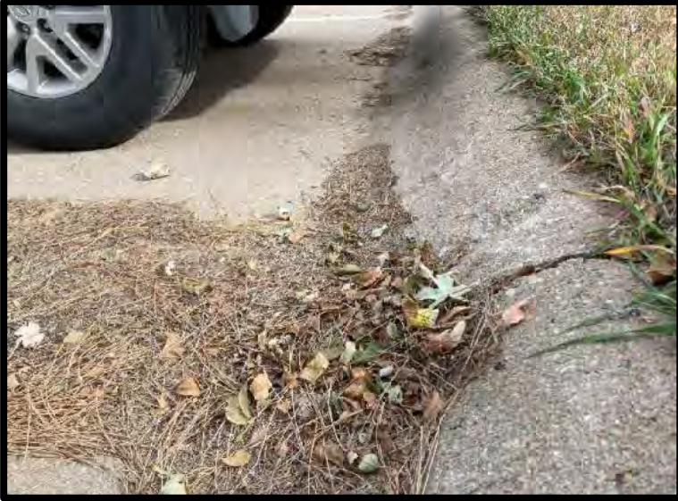
Picture 1: Debris in Curb Line Employee Parking – 11/14/2023
