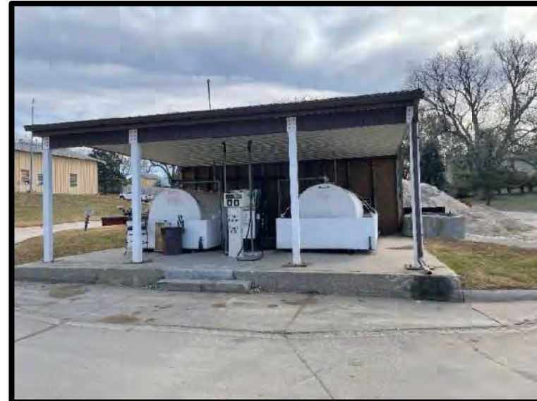
Picture 24: Covered Fueling Area – 11/14/2023
