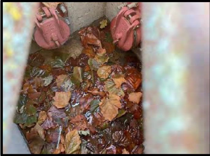
Picture 13: Area Inlet Southwest of Pool – 11/21/2023
