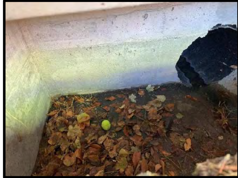
Picture 12: Inlet at Main Facility Entrance – 11/21/2023
