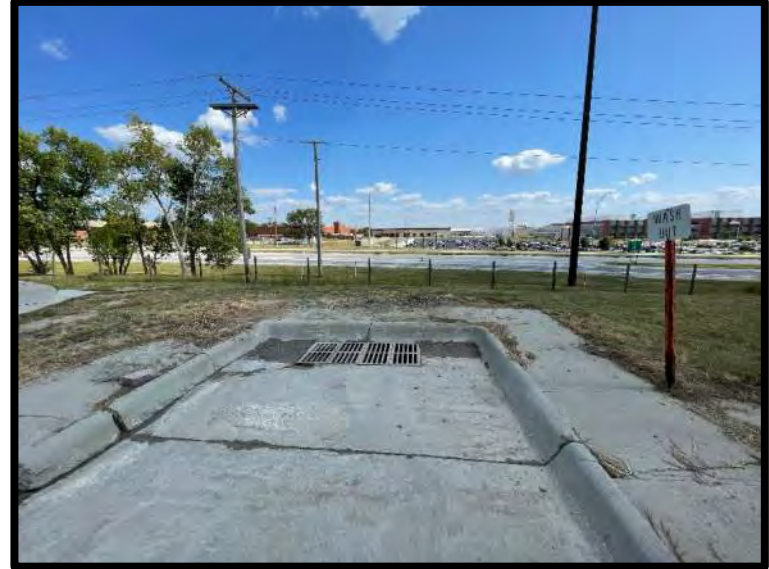
Picture 2: Washout Area – 9/14/2023
