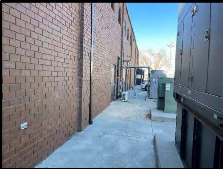
Picture 7: Downspout Diverted to Pervious Surface – 11/21/2023
