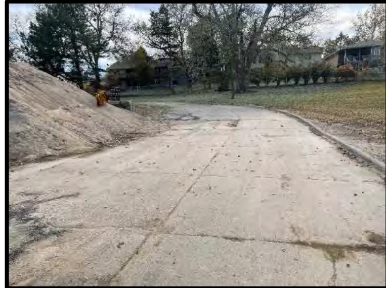
Picture 32: Pavement West of Sand Storage – 11/14/2023
