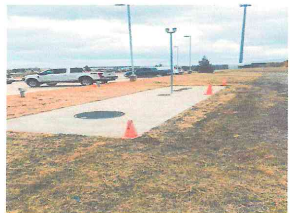
Photo #18: Underground Fuel Storage Tak
