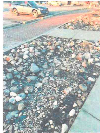
Photo #20: Administration Parking Lot East Drainage System-Additional Photo
