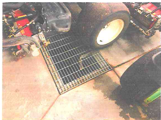
Photo #10: Floor drain in maintenance shop connected to sanitary sewer.
