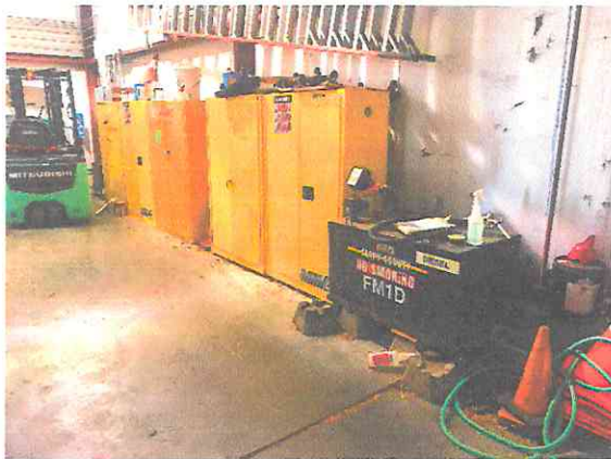
Photo #5: Hazardous material storage cabinets are in good working condition. Double-walled Diesel tank in good working condition.
