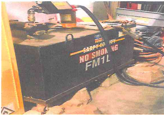
Photo #3: 100 Gallon Bulk Diesel Storage - Double Wall Tank
