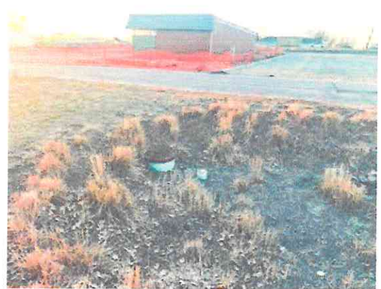
Photo #16: Ground drain basin for East Driveway
