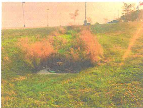
Photo #22: Small Bioretention Cell #1 taking Drainage from North Parking Area.
