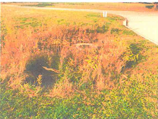
Photo #23: Small Bioretention cell #2 taking Drainage from North Parking Area.
