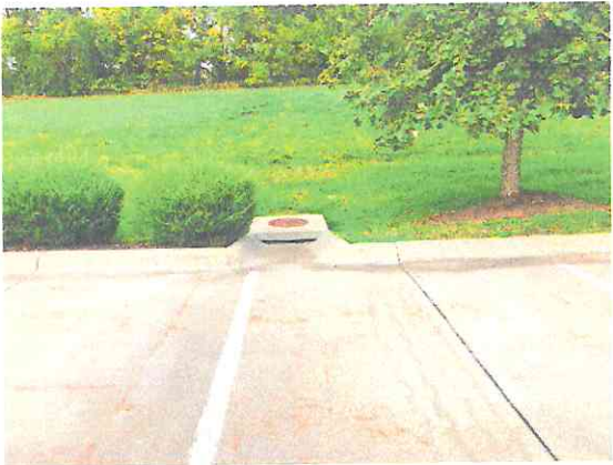
Photo #14: Storm drain inlet (north), west parking
