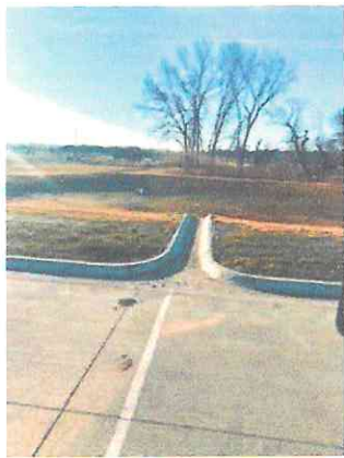
Photo #9: Drainage swale leading from south parking area to detention basin. Monitor for any erosion and conduct necessary repairs.
