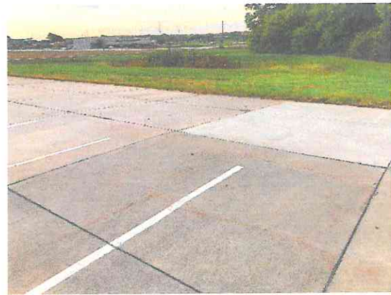
Photo #10: South parking area drains toward the detention basin, south side of property.
