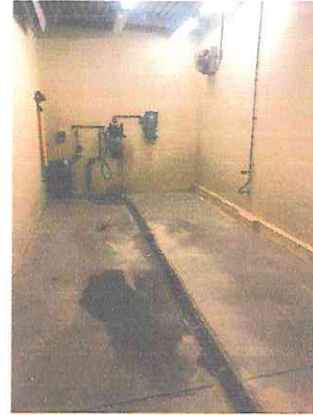
Photo #8: Vehicle Wash Bay - Floor Drain Tied to Sanitary Sewer with a Catch Basin.
