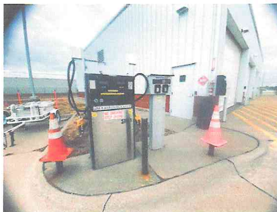
Photo #20: Fuel Station
