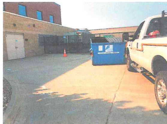
Photo #12: HVAC units and solid waste dumpster on north side of building
