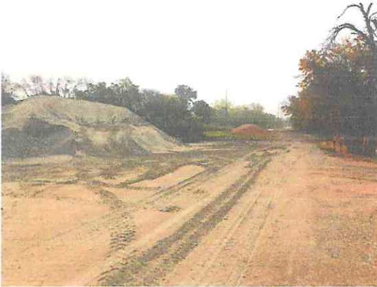
Photo #1: Stockpiles located on north edge of facility property, looking east towards entrance.
