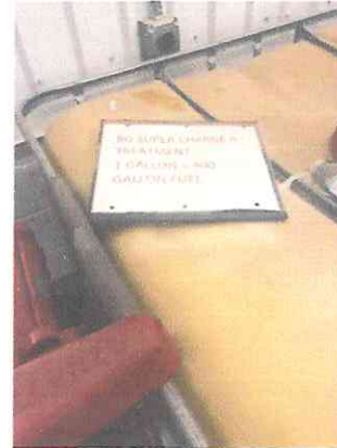
Photo #2: Fuel Treatment Label on Bulk Tank, Cold Storage Building.
