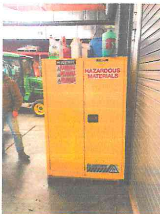
Photo #11: Hazardous materials cabinet for gasoline and gas mix cans.
