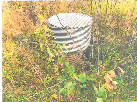
Photo #8: Detention basin outlet riser pipe. Annual maintenance should include ensuring outlet structure is clear of debris and excess vegetation.
