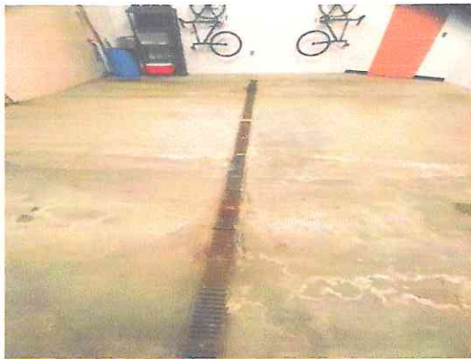
Photo #3 Garage Floor Drain - Sally Port
