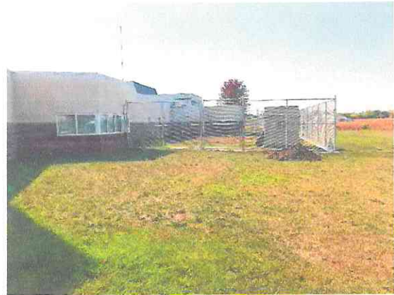
Photo #2 New fencing installed. Roof drain extension will be modified to accommodate drainage beyond the fence.
