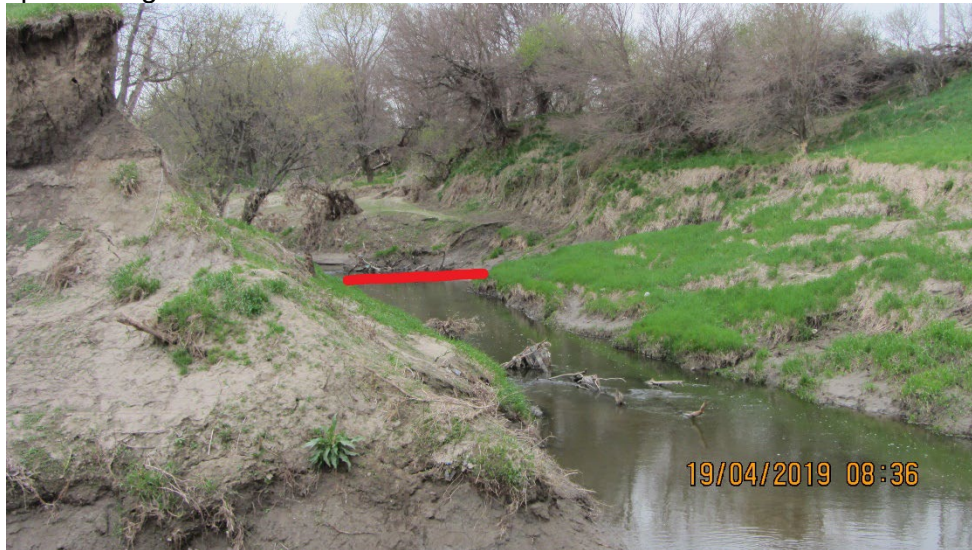
Figure 2. Exposed sewer line on West Papillion Creek just above confluence with South Papillion Creek (looking upstream from the confluence). Pipe location highlighted.
