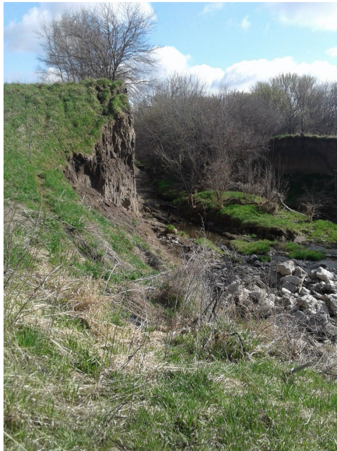
Figure 13. Bank erosion below the culvert structure on Giles Rd. near 180 th St.
