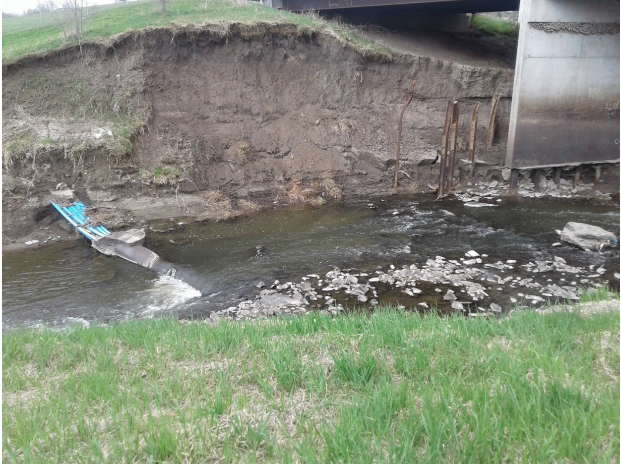
Figure 15. Bank erosion caused by channel degradation and surface water discharge into channel perpendicular to bank. Note telecom lines exposed by erosion.
