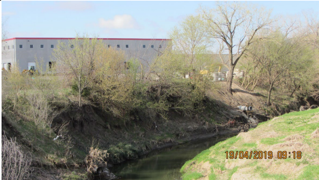
Figure 5. Right bank erosion above the Giles Road Bridge (looking upstream)
