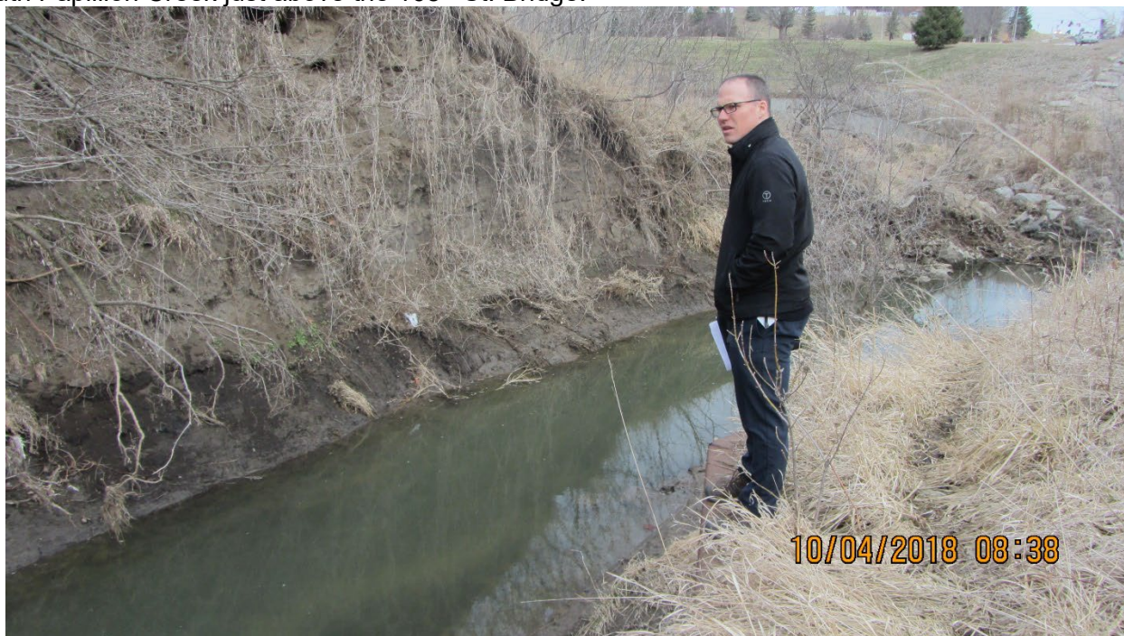
Figure 8. Channel incision upstream of 168 th St. Bridge
