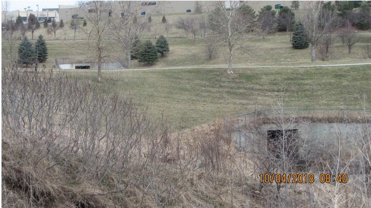
Figure 9. NRCS designed neighborhood runoff detention structure
