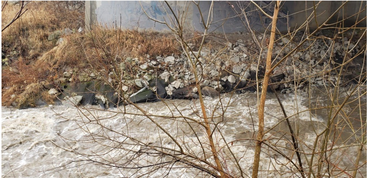
Figure 8-6: FG Reach 2b –South Papillion Creek: Existing Riprap Forming GCS Under South 126 th Street Bridge
