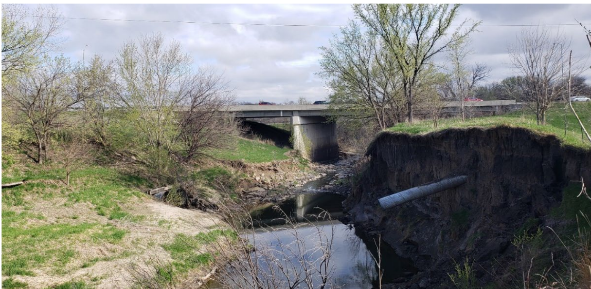
Figure 4-60: South Papillion Creek Upstream of Giles Road Bridge Showing Right Bank Erosion of Culvert Outlet
