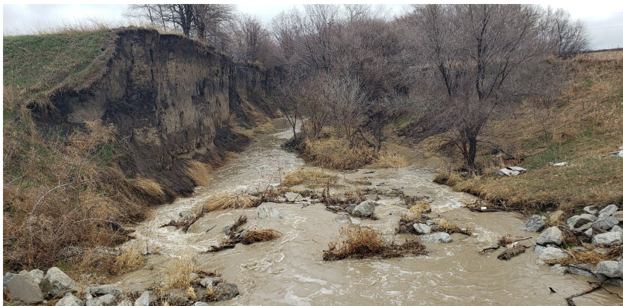
Figure 8-12: FG Reach 6, South Papillion Creek – Downstream of Giles Road Culverts Showing Local Channel Degradation at Culvert Outlets and Unstable Banks Downstream
