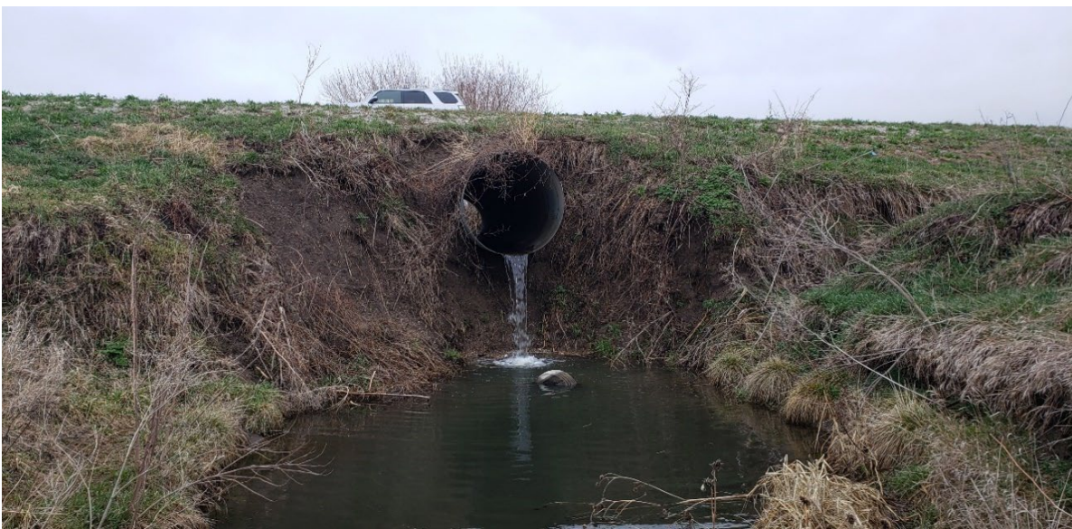
Figure 8-5: South Papillion Creek FG, Reach 9 – Downstream Terminus of Reach 9, Illustrating a Perched Culvert at South 216 th Street
