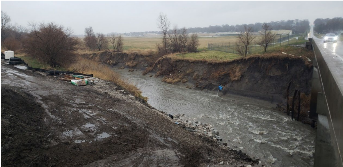
Figure 7-2: FG Reach 5 – Right Bank Erosion Downstream of 132 nd Street Bridge, West Papillion Creek
