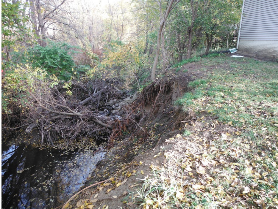
Figure 6-6: EWN LPSTP Pre-project Conditions – Bank Erosion on Left Bank Threatening Residence, Bettendorf, Iowa
