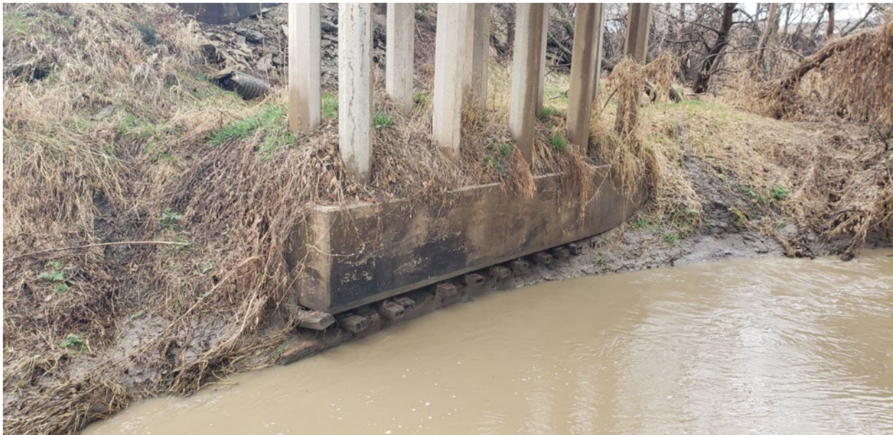
Figure 8-14: FG Reach 6, South Papillion Creek – Railroad Bridge in Upstream Section of Reach Showing Scour and Potential Undercutting of the Wood Footings
