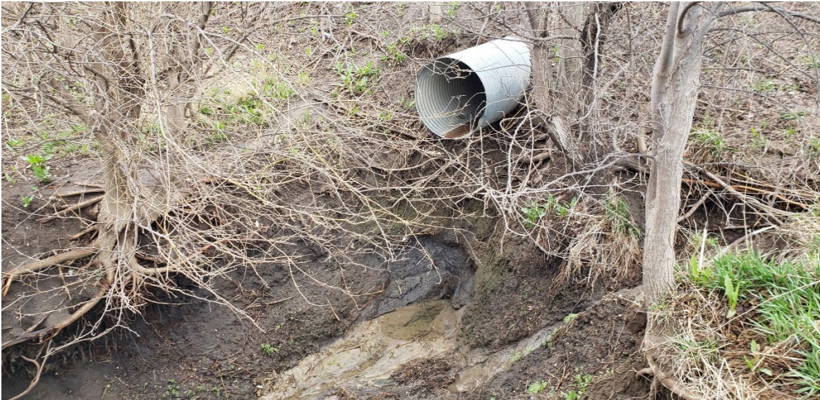
Figure 8-4: South Papillion Creek FG, Reach 9 – Perched Culvert at Harrison Street, Upstream End of Reach 9
