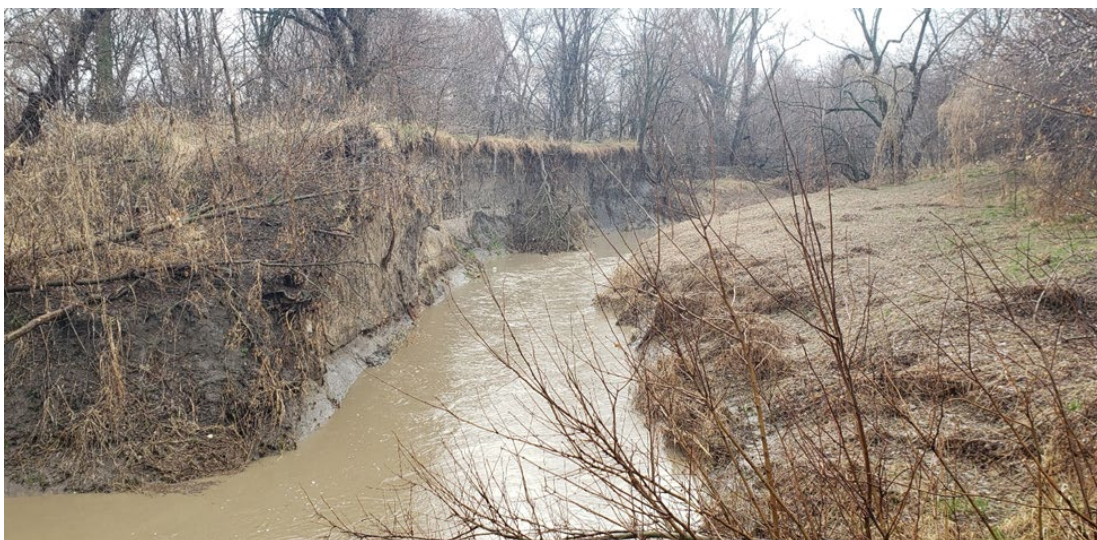
Figure 8-15: FG Reach 4, South Papillion Creek – Channel Section Immediately West of South 167 th Court Showing Vertical Right Banks in a Meandering Incised Channel
